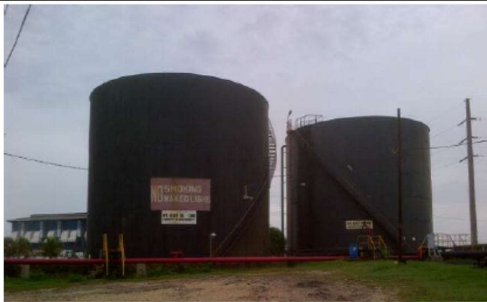
Photo 7 – HFO Tank #1 and 2
