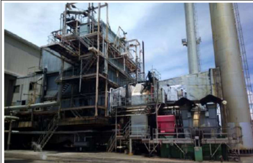
Photo 6 - A section of a boiler
