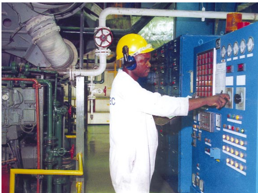
A technician dispatches power in the engine room at Cul-de-Sac
